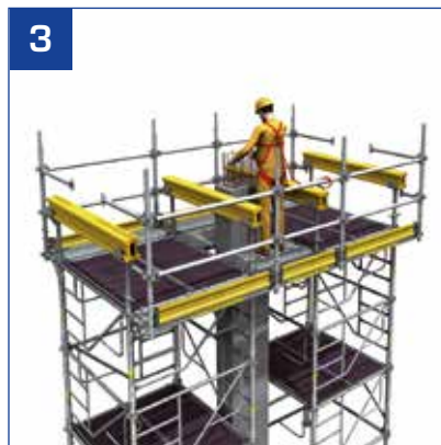
- Reinstall the planks with trapdoors. The operator must use a fall prevention system until the concrete beams have been installed.
