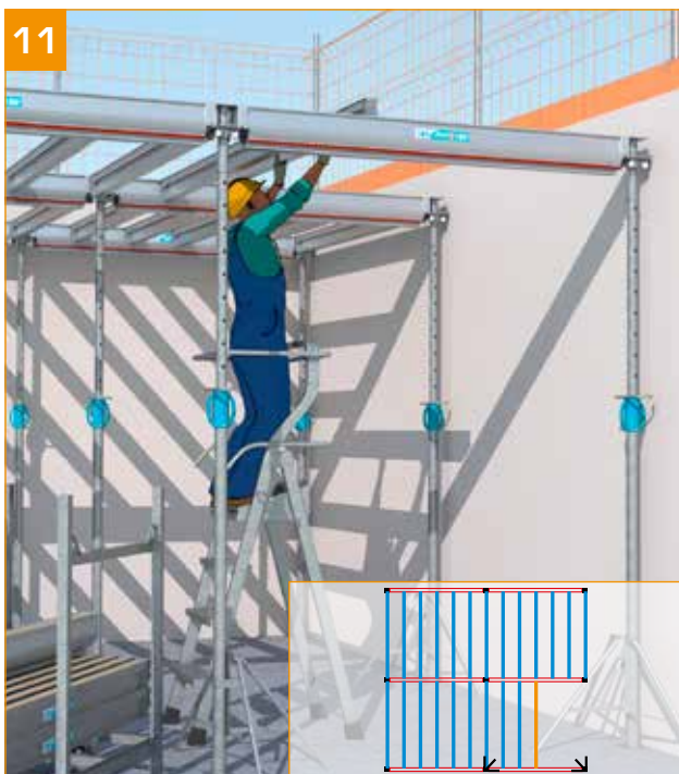
- Move the secondary beams forwards from one to the next, keeping a gap of 39 cm.
